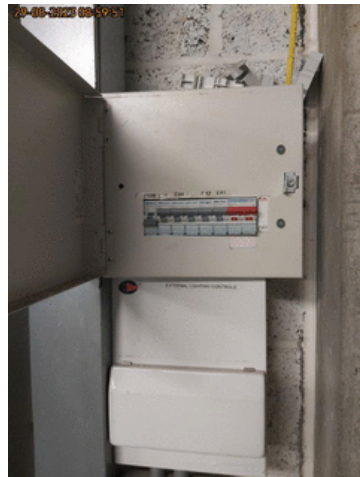
Distribution Board Photo 5
