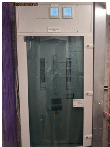
Distribution Board Photo 9
