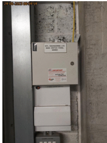
Distribution Board Photo 6
