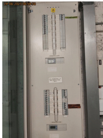
Distribution Board Photo 4
