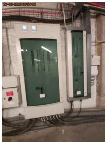
Distribution Board Photo 2
