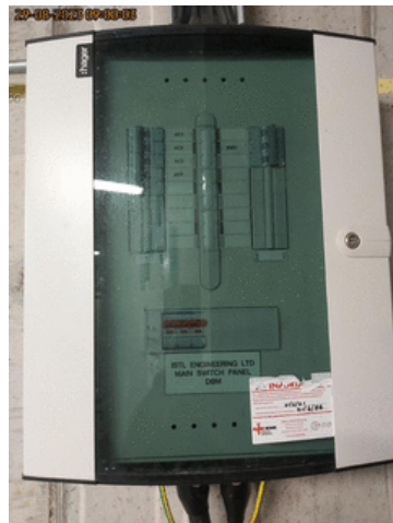
Distribution Board Photo 7
