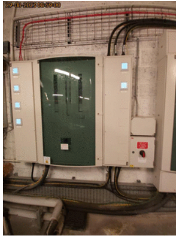
Incoming Supply Photo 1
