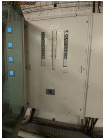
Distribution Board Photo 1
