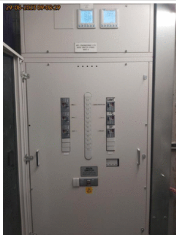
Distribution Board Photo 10
